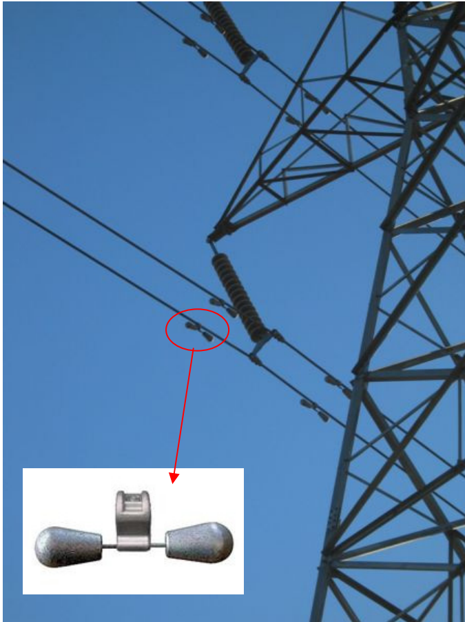
Vibration absorber in the transmission lines
